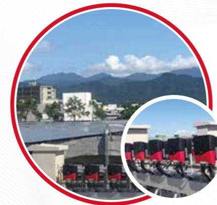
TAOYUAN CITY, TAIWAN 5MW
